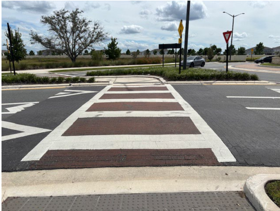
Photo 20 - Deteriorating Thermoplastic and Worn Coloration
