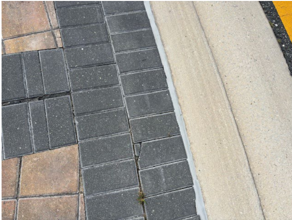
Photo 7 - Broken Concrete Pavers on Truck Apron
