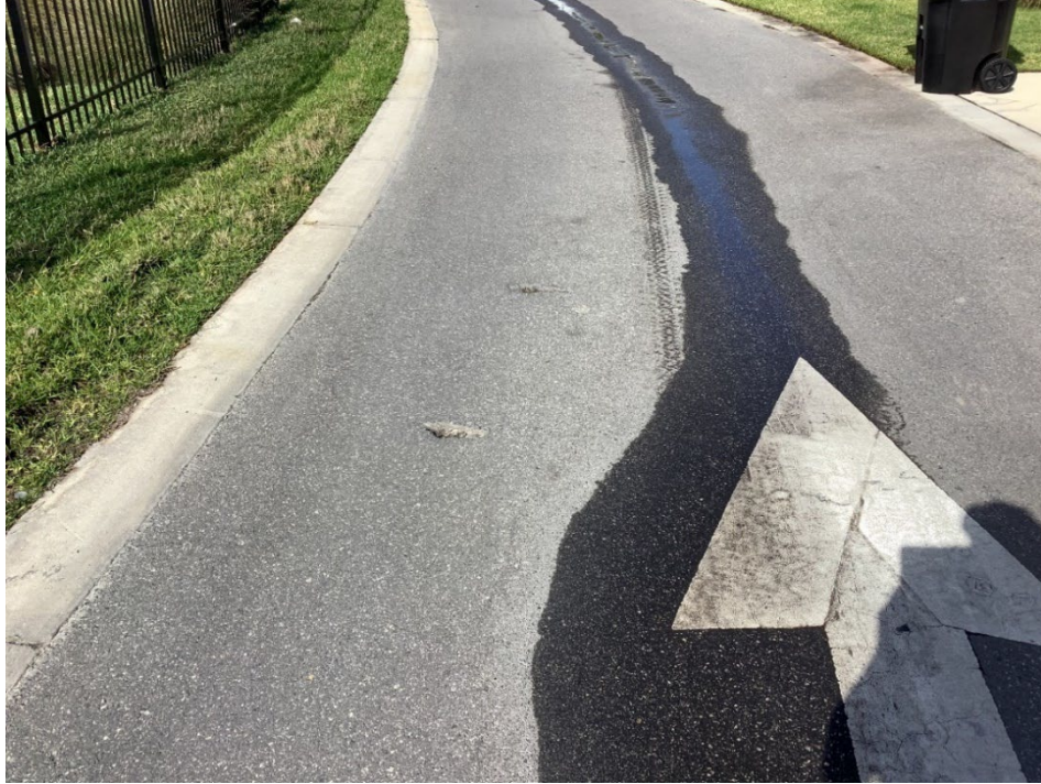
Photo 14 - Laggett Alley – Asphalt Damage (No Observed Changes) (Refer to Prior Photo 28 – 2025 Assessment)
