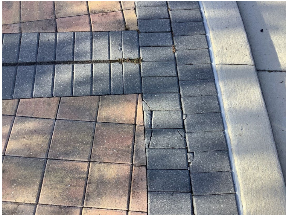
Photo 5 - Broken Concrete Pavers on Truck Apron (Increased Damage Observed) (Refer to Prior Photo 8 – 2025 Assessment)
