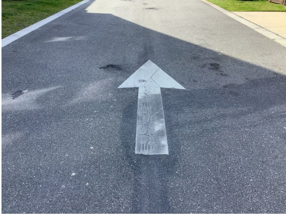
Photo 12 - Laggett Alley – Asphalt Damage (No Observed Changes) (Refer to Prior Photo 26 – 2025 Assessment)
