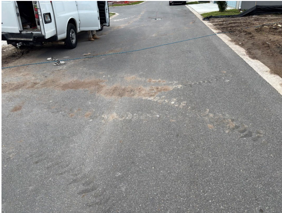
Photo 18 - Fiddley Alley – Asphalt Damage (New Alley - New Photo – 2026 Assessment)
