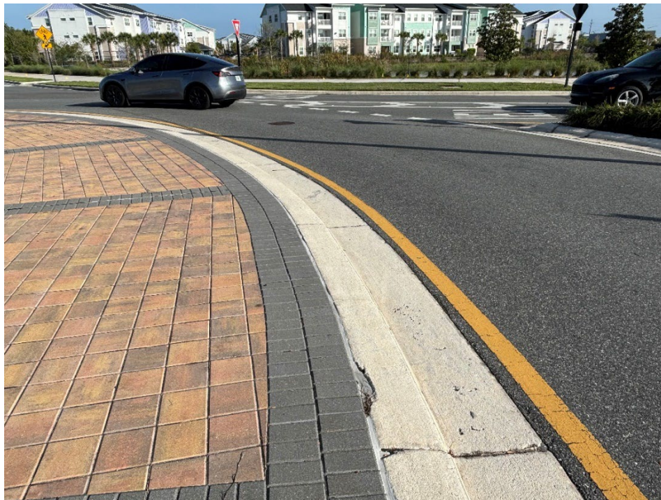
Photo 10.1 - Damage to Concrete Curb Along Truck Apron (New Photo – 2026 Assessment)
