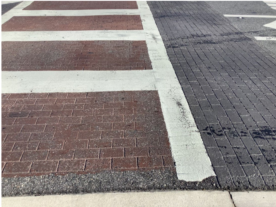
Photo 9 - Deteriorating Thermoplastic and Worn Coloration (No Observed Changes) (Refer to Prior Photo 15 – 2025 Assessment)
