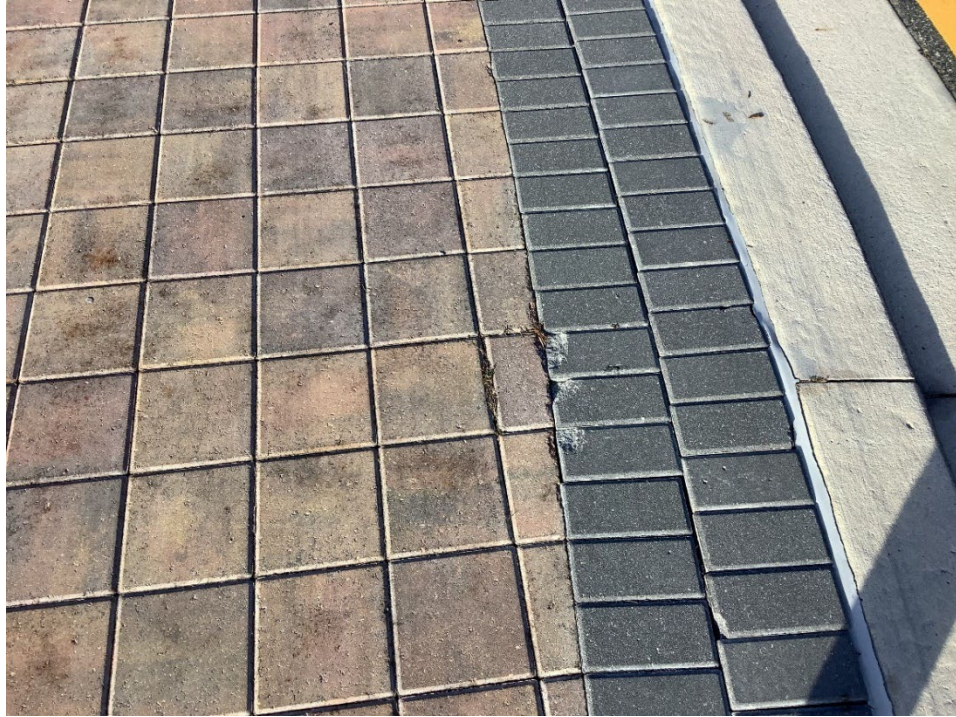
Photo 4 - Broken Concrete Pavers on Truck Apron (No Observed Changes) (Refer to Prior Photo 6 – 2025 Assessment)
