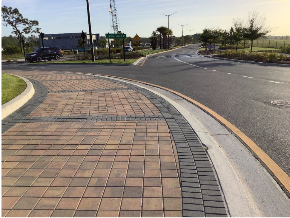
Photo 1 - Damage to Concrete Curb Along Truck Apron (No Observed Changes) (Refer to Prior Photo 1 – 2025 Assessment)
