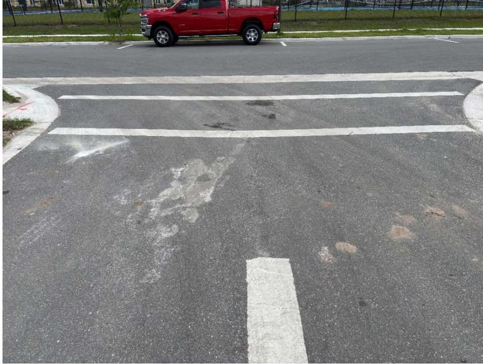
Photo 19 - Fiddley Alley – Concrete Spilled into Asphalt (New Alley - New Photo – 2026 Assessment)
