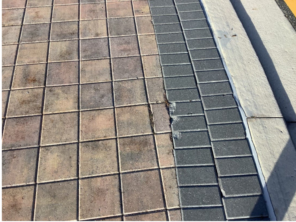
Photo 4 - Broken Concrete Pavers on Truck Apron (No Observed Changes) (Refer to Prior Photo 6 – 2025 Assessment)
