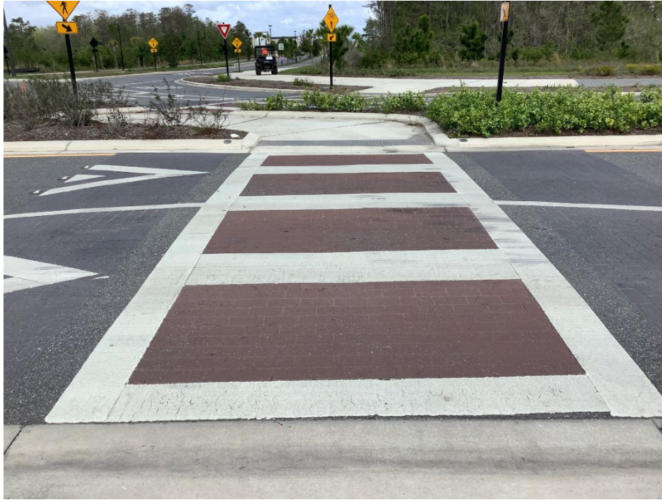
Photo 3 - Deterioration of Thermoplastic and Worn Coloration (No Observed Changes) (Refer to Prior Photo 5 – 2025 Assessment)
