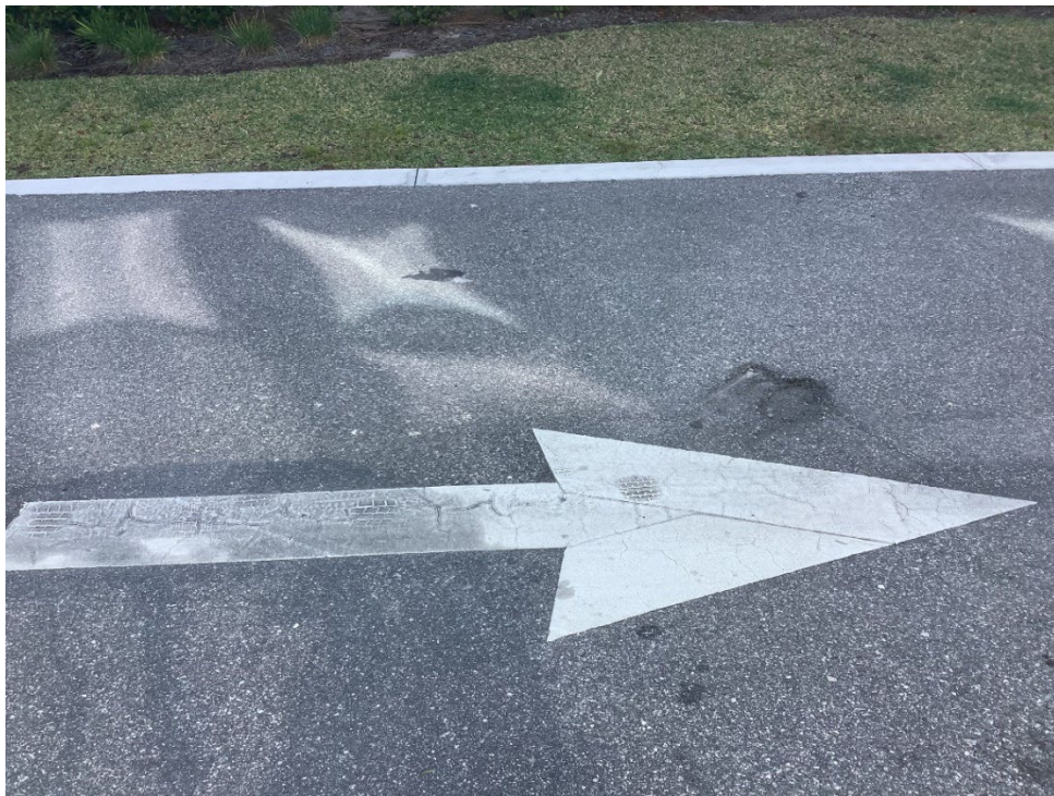
Photo 13- Laggett Alley – Asphalt Damage (No Observed Changes) (Refer to Prior Photo 27 – 2025 Assessment)
