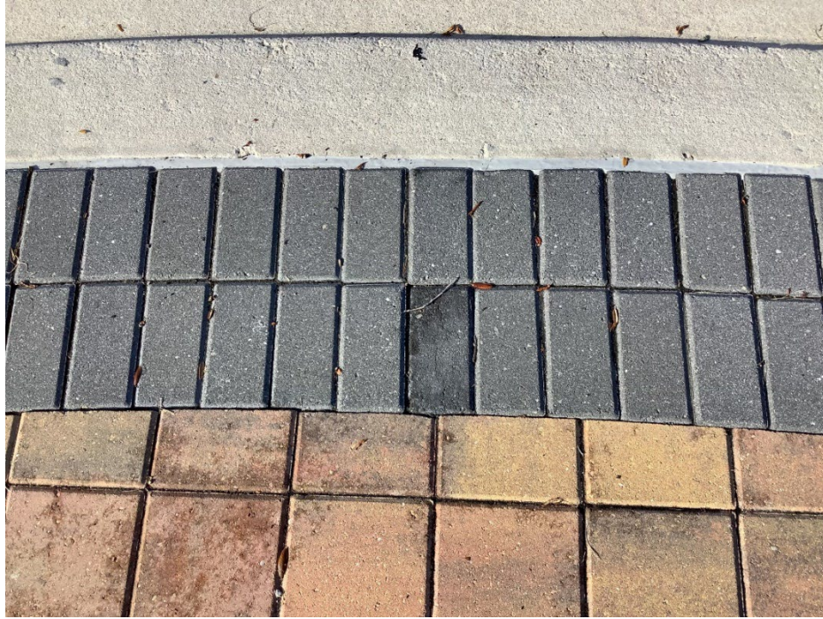
Photo 10 - Uneven Concrete Pavers on Truck Apron (No Observed Changes) (Refer to Prior Photo 18 – 2025 Assessment)
