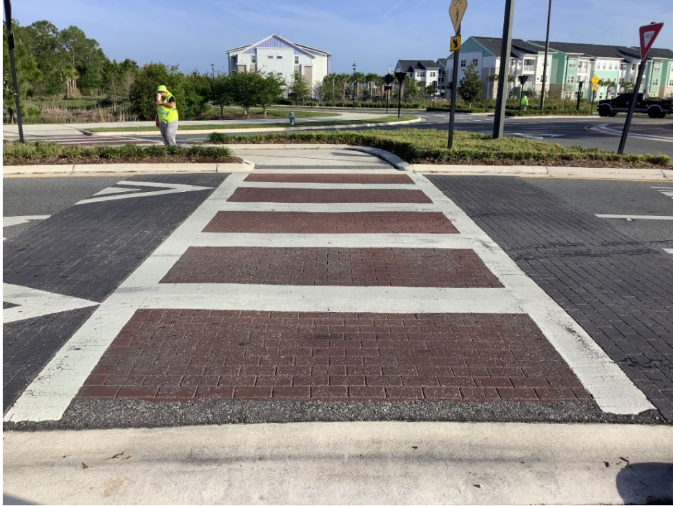
Photo 8 - Deteriorating Thermoplastic and Worn Coloration (No Observed Changes) (Refer to Prior Photo 14 – 2025 Assessment)
