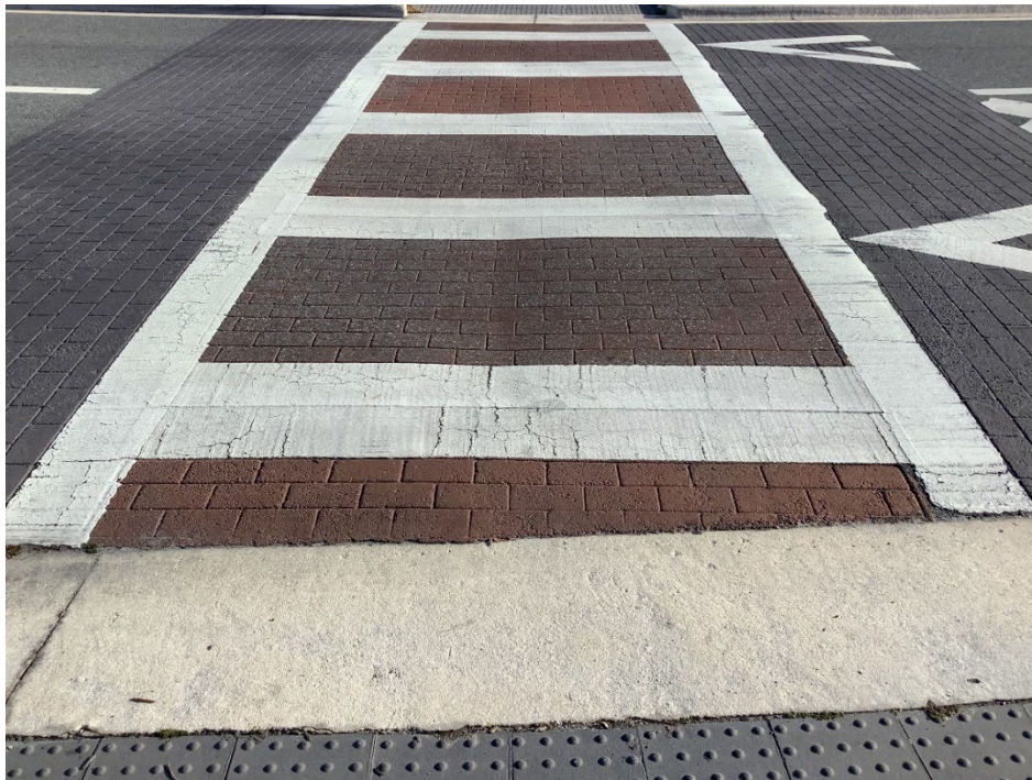
Photo 7 Deteriorating Thermoplastic and Worn Coloration (Further Deterioration Observed) (Refer to Prior Photo 13 – 2025 Assessment)
