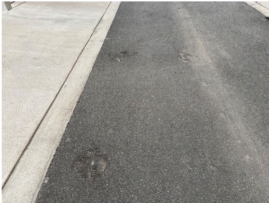
Photo 22 - Ganzel Alley – Asphalt Raveling (New Alley - New Photo – 2026 Assessment)
