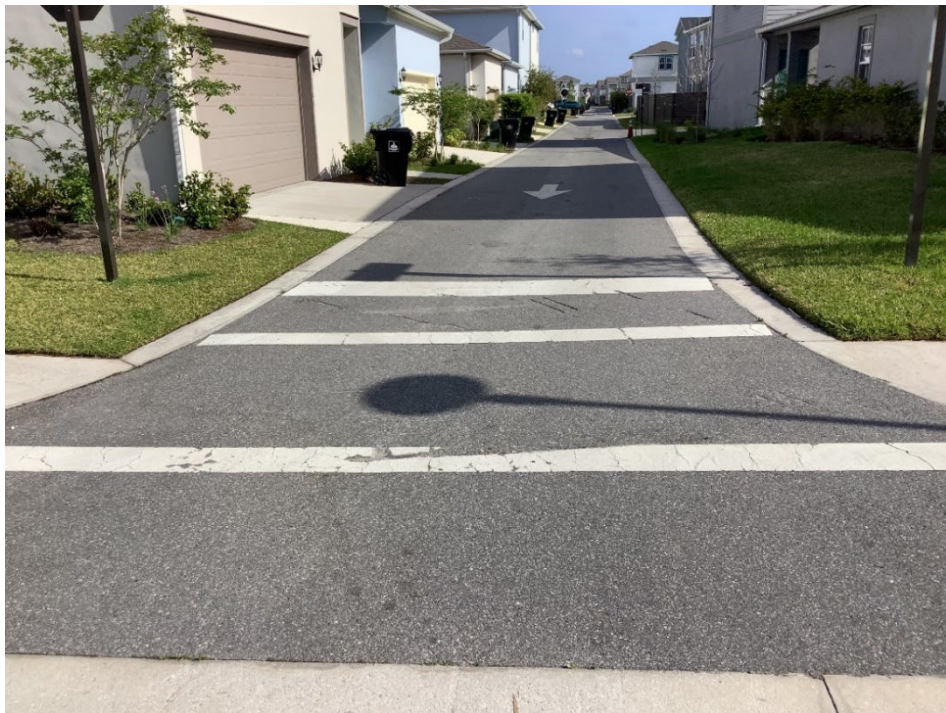
Photo 15 - Marconi Alley – Deterioration of Thermoplastic and Gouged Asphalt (No Observed Changes) (Refer to Prior Photo 30 – 2025 Assessment)
