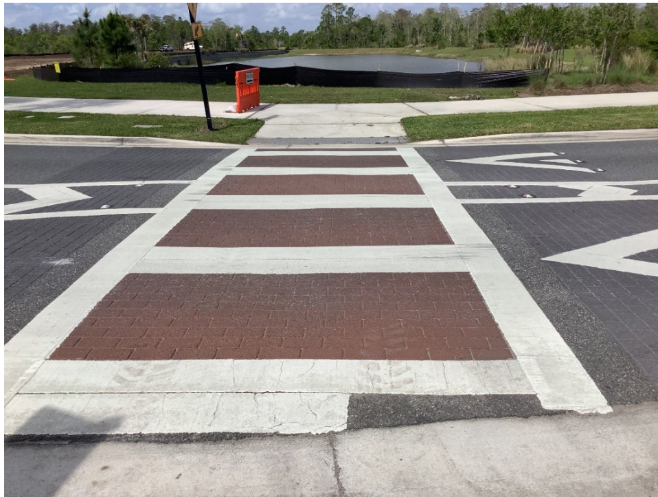
Photo 2 - Deterioration of Thermoplastic and Worn Coloration (No Observed Changes) (Refer to Prior Photo 4 – 2025 Assessment)
