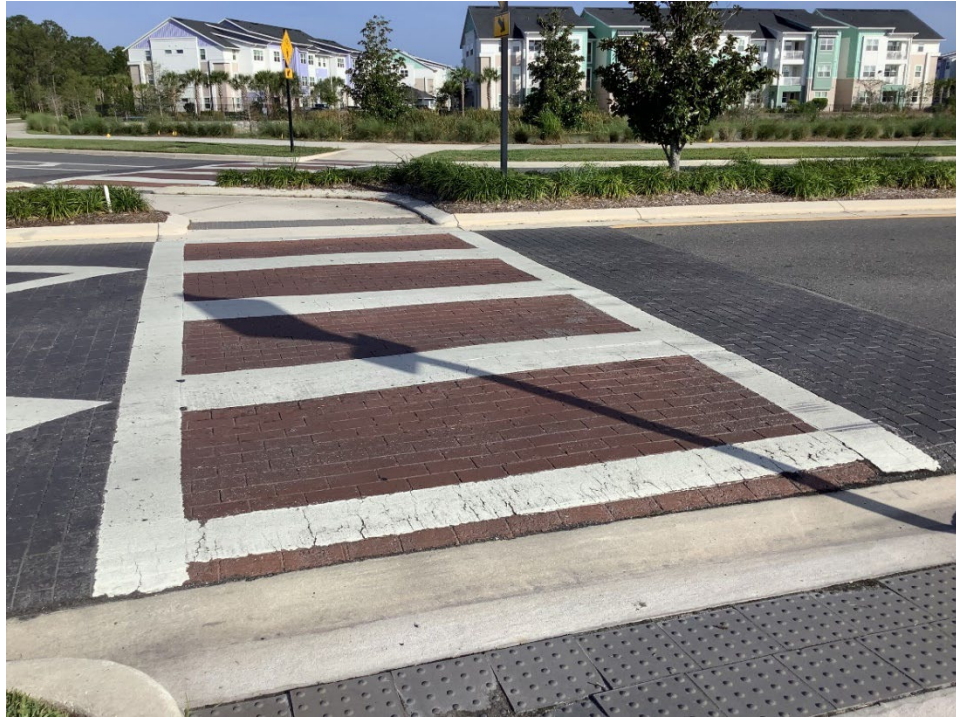
Photo 11 Deteriorating Thermoplastic and Worn Coloration (Further Deterioration Observed) (Refer to Prior Photo 21 – 2025 Assessment)
