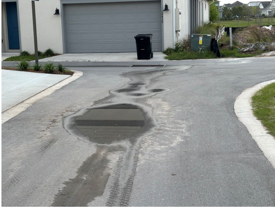
Photo 17 - Rostand Alley – Low Spot In Valley (New Alley - New Photo – 2026 Assessment)
