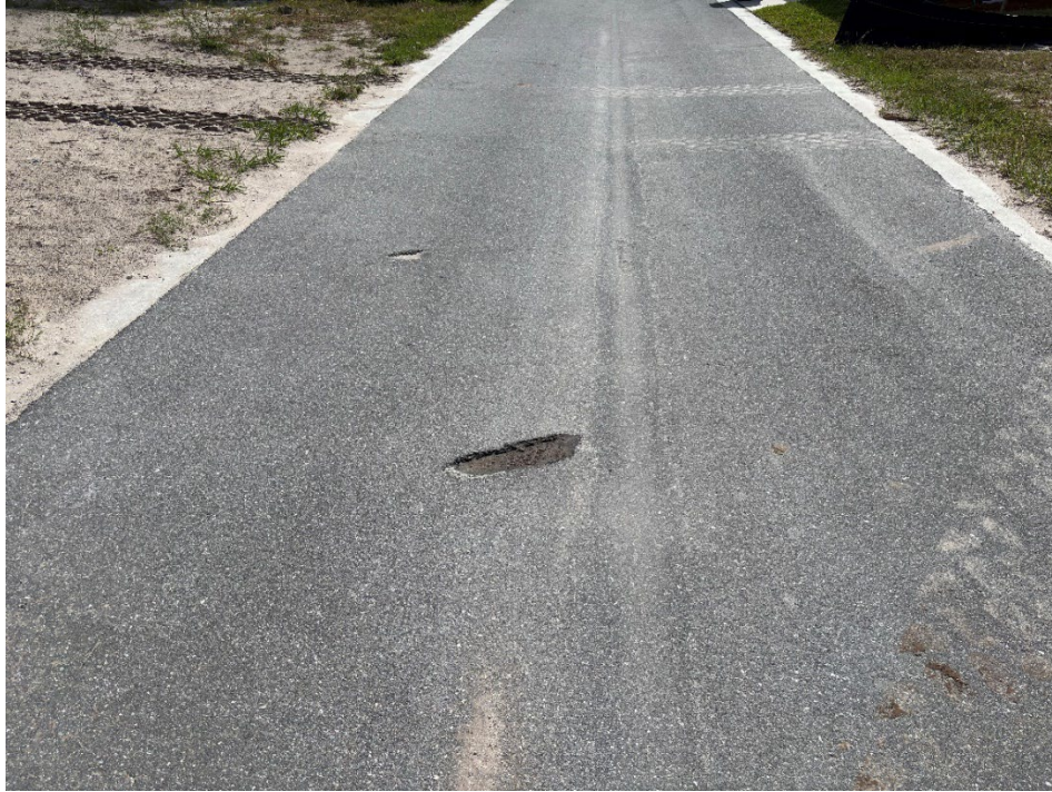
Photo 21 - Hasselmann Alley – Asphalt Damage (New Alley - New Photo – 2026 Assessment)
