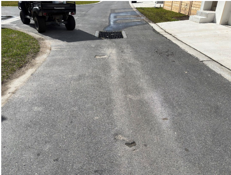
Photo 20 - Gobat Alley – Asphalt Damage (New Alley - New Photo – 2026 Assessment)
